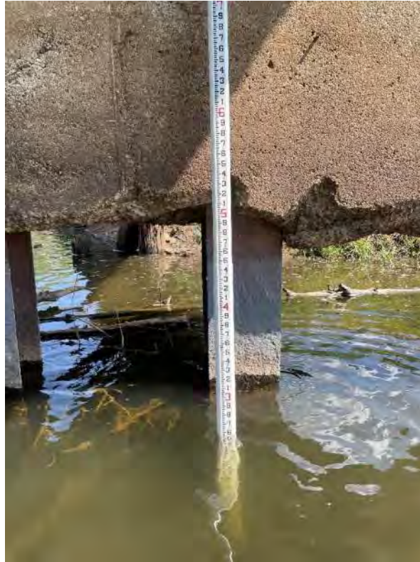
Photo 8: Five feet of scour under railroad bridge piers
