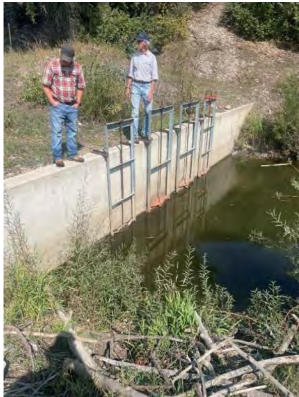
Photo 3: Control gates for water delivery
