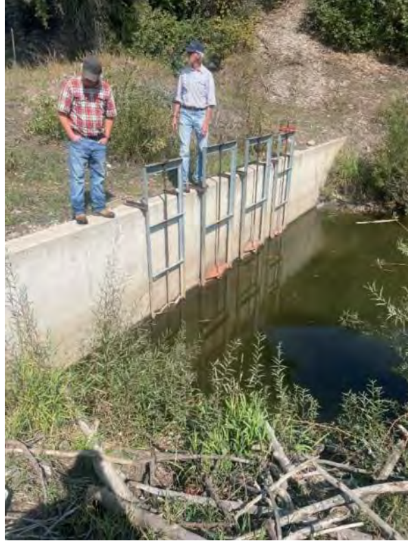
Photo 3: Control Gates for Water Delivery
